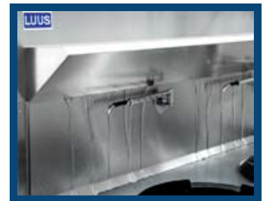
Water Cooling System
